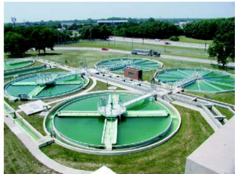
Fig. 21.9: Sewerage treatment plant
