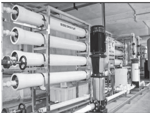
Figure 3.13: Membrane module used in commercial plant
