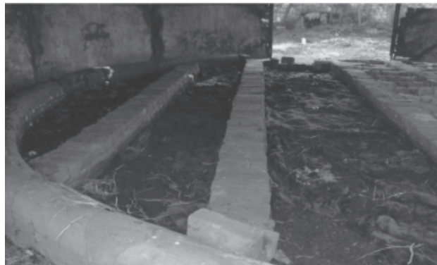
Fig. 3.5: Composting in Cemented Vermikomposting Pit
