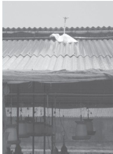
Fig. 5.28: Sprinkler on the roof top
